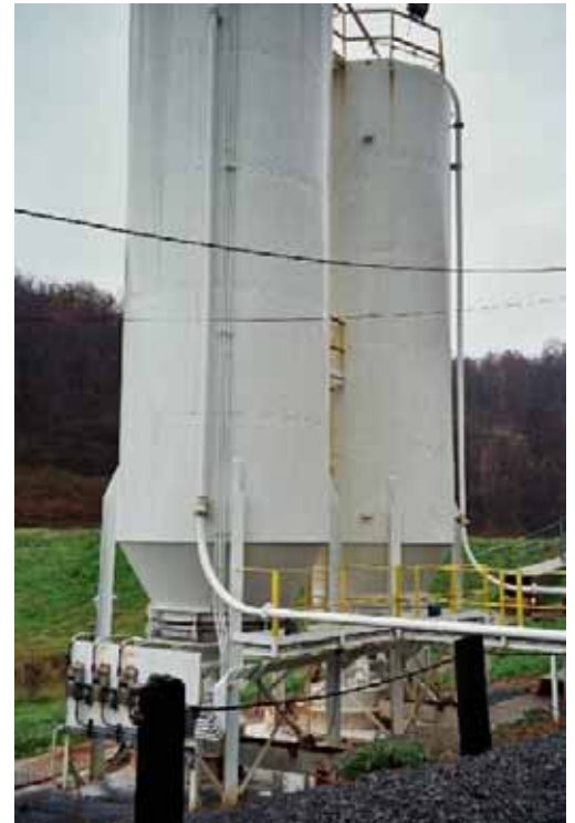
Figure 1: Active treatment system.
