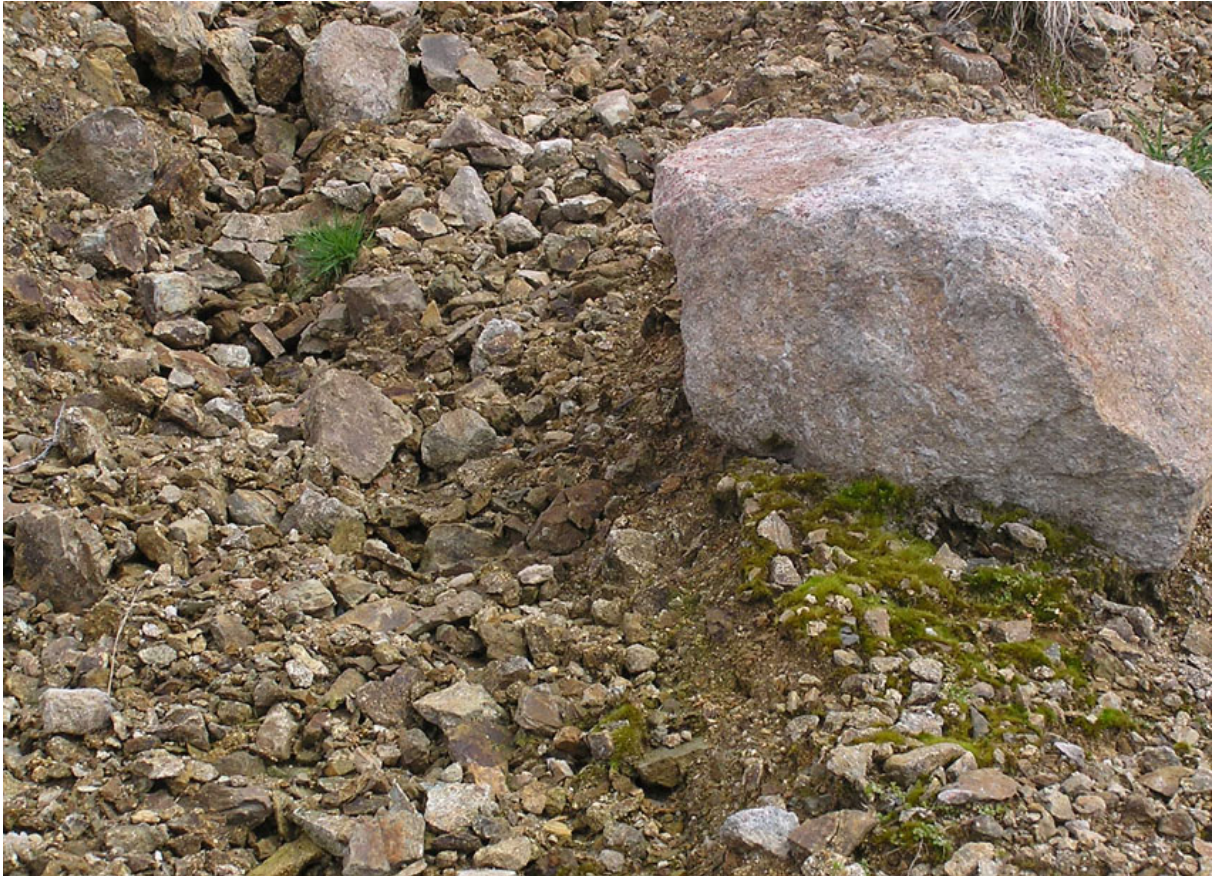
Figure 4. Erosion runnel on the granite veneer site with adjacent moss growing in the protection provided by a large boulder.
